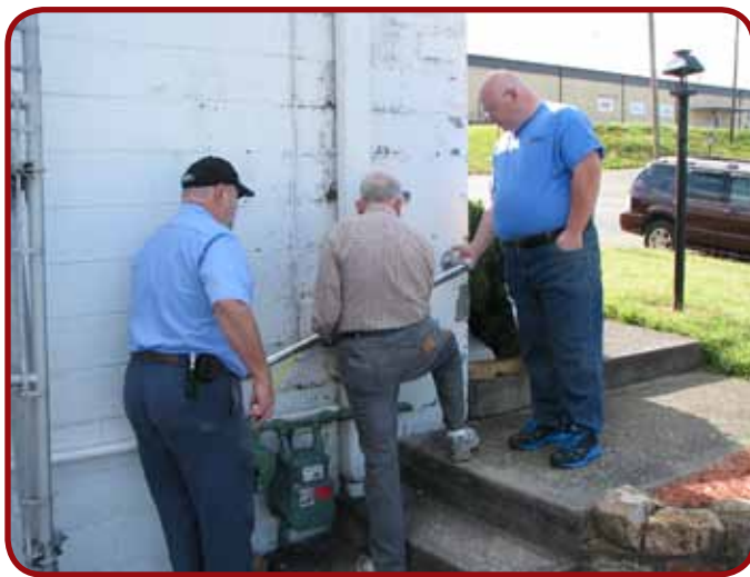
Ben Shank, Gordon Hamilton and Joe Shaw spent part of their time at the September 2013 Archives work session installing a hand-rail for the steps leading into the NWHS building. Alex Schust photo
